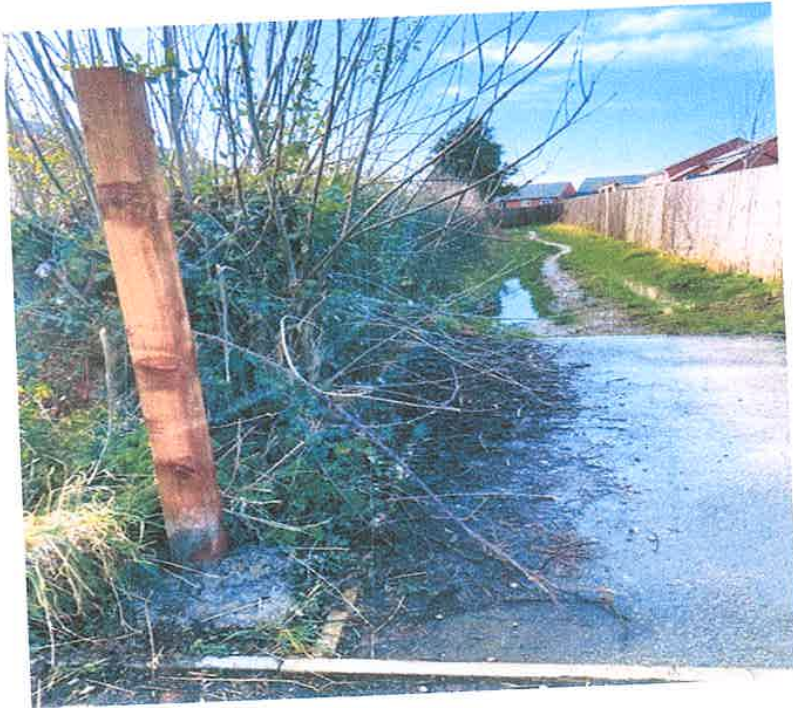
IMAGE 15: TRACK – Viewed from behind Substation (ESS) on Shearwater road looking towards Churton Road. Photograph shows new erected fence and recent access on foot evident February 2020
